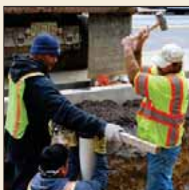
Steve Shofar (center), Chief of Montgomery County's Watershed Management Division, is helping to direct the $305 million effort. The Maryland county is hiring about 3,300 workers to improve its stormwater control systems. The workers include Marcus Irving (below, left).
